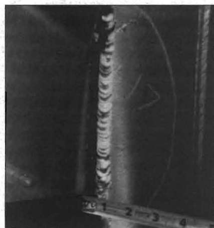
FIG. 7: Detail of failed diaphragm connection.
