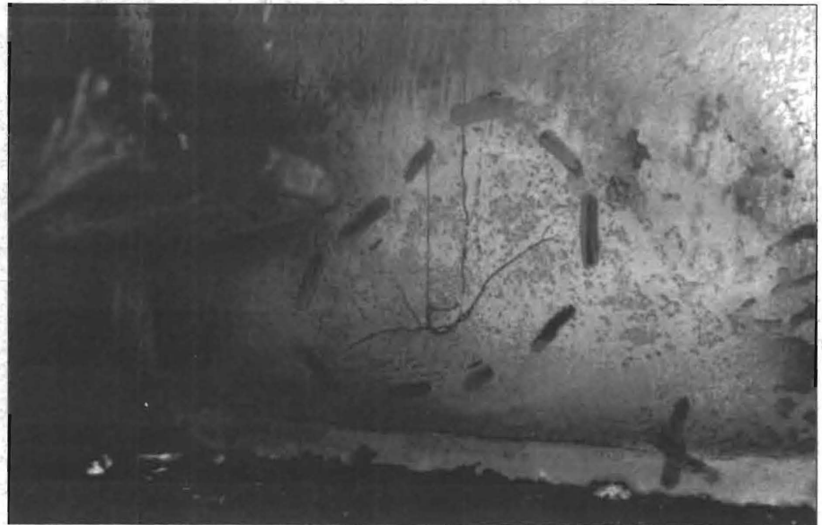
FIGURE 2: Example of fatigue cracking around connection plates and the welds on the bridges.
