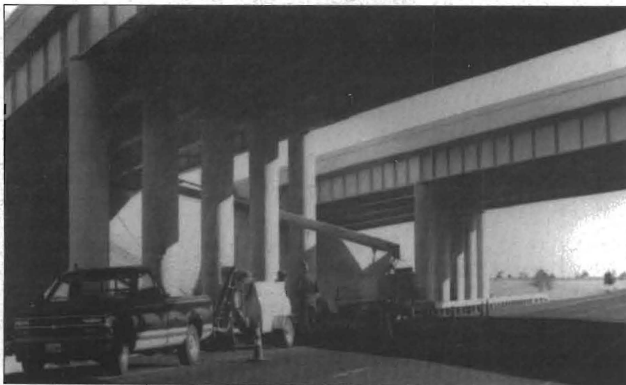
FIGURE 1: Researchers and TxDOT staff prepare the IH-20 Midland County bridges for testing.
