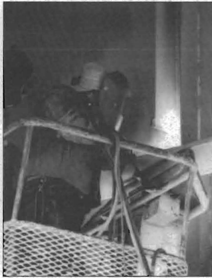
FIG. 11: Repair types 1 and 2 required welding equipment for air arc gouging and flame cutting respectively.
