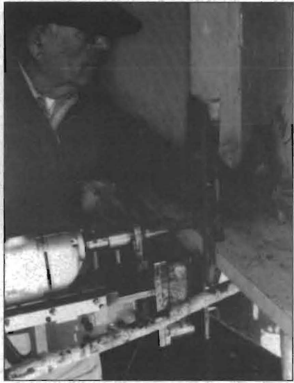
FIG. 10: Both ends of toe weld cracks were drilled in all three types of repairs.
