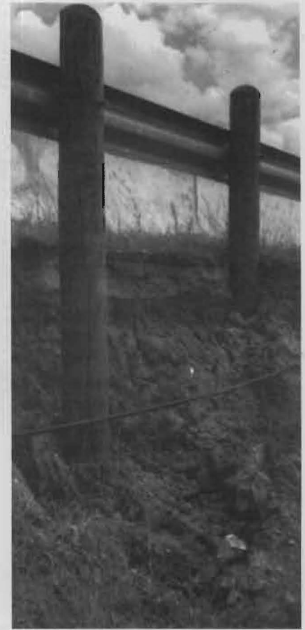
FIG. 2B: Closeup showing erosion.
