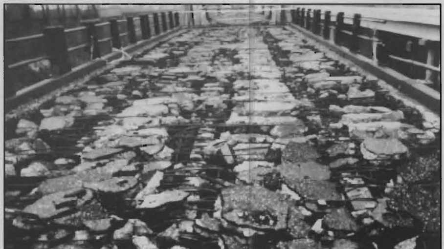
FIG. 1: Eastern Texas deck replacement due to severe corrosion of uncoated rebar. Epoxy-coated steel, at a slightly higher initial cost, might have added 20 years of useful life.
