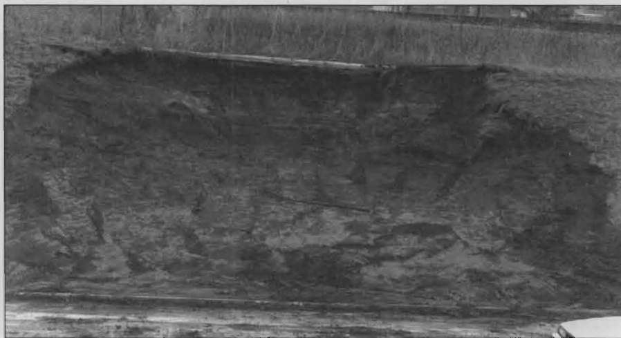
FIGURE 1: Excavated slide area.
