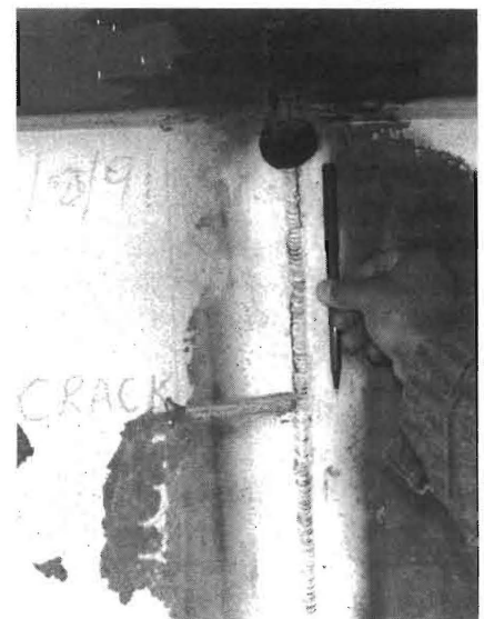
FIGURE 9: BRINSAP inspector documenting a crack.
