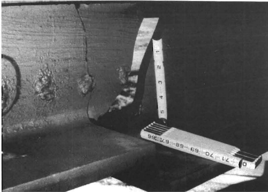
FIGURE 6: Fracture at weld-filled holes [Ref. 6].
