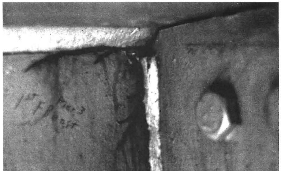
FIGURE 7: Cracking in a girder web at a floor beam connection plate which was not welded to the top flange. (Courtesy of Dr. John Fisher, Lehigh University.)
