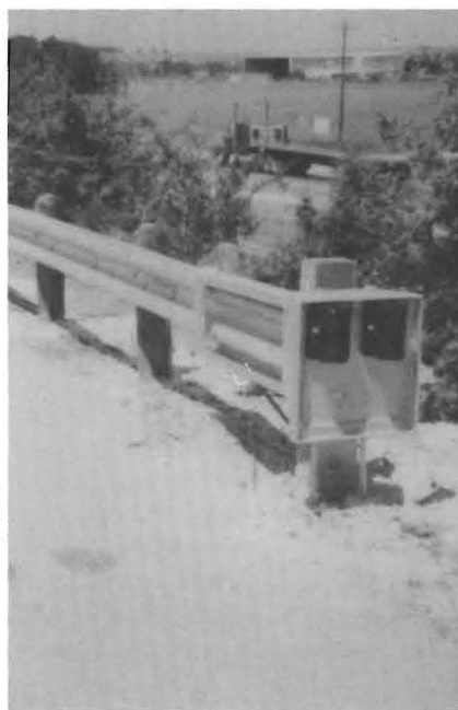
FIG. 1: First installation of Study 404 guardrail end, Austin, IH-35, 21 June 1990.
