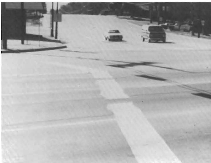
FIGURE 1: Intersection showing typical distress.
