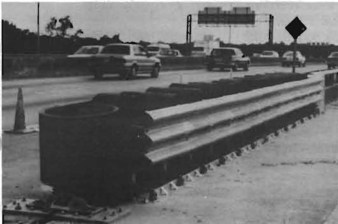
FIG. 1: Low-maintenance crash attenuator.
