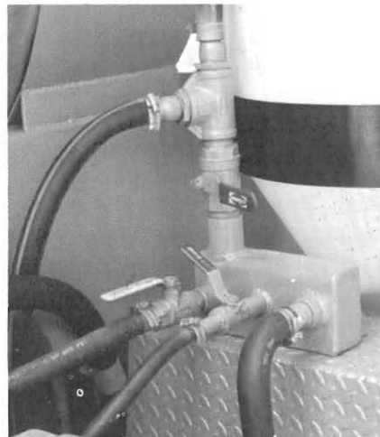
FIGURE 8 Bypass manifold; bypass valve in upper right.
