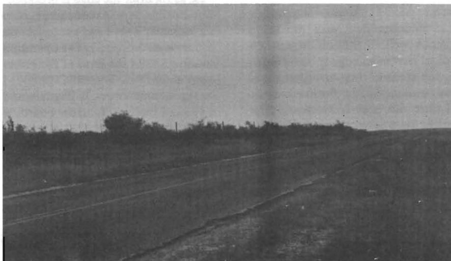
FIGURE 2 A broken pavement edge.
