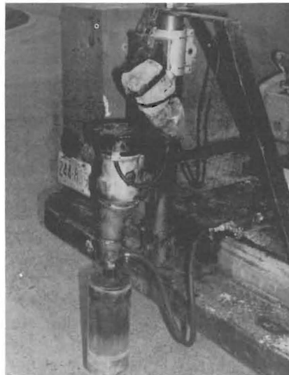
FIG.4 Detail of the water valve.
