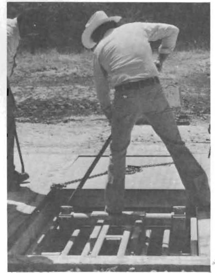
FIG. 3 Installing the axle and wheel (AX/WHL) reference scale.
