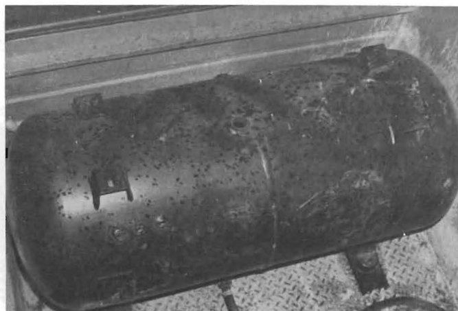
FIGURE 7 50 gallon water tank.
