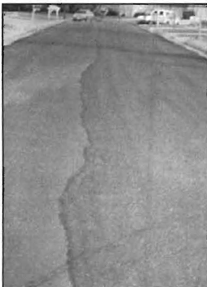
FIG. 3: A bad longitudinal joint. Joints should be straight and even.
