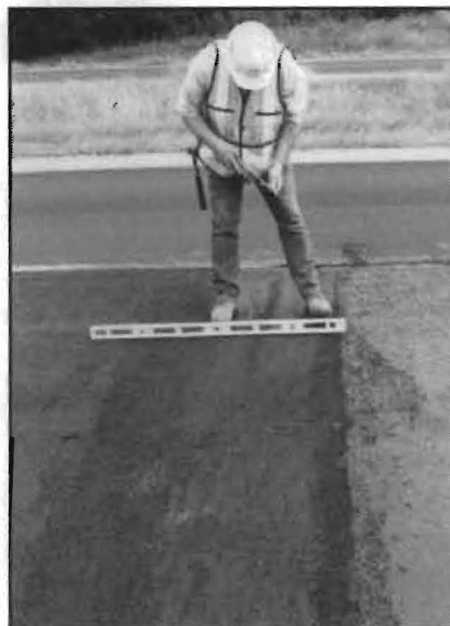
FIG. 4: A bad transverse joint. Note the irregular-looking surface.
