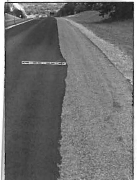
FIG. 5: A bad edge. Like longitudinal joints, edgelines should be straight.
