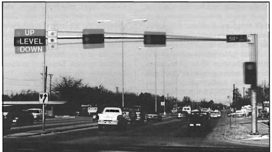
FIG. 1: An in-service traffic signal structure exhibiting galloping. Photo composite by Michael Gray, Center for Transportation Research.
