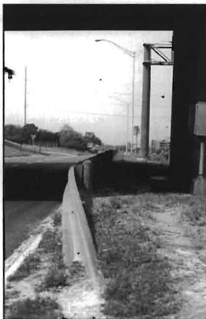
FIG. 1: This guardrail system protects vehicle from concrete columns and, further afield, from an overhead sign structure.
