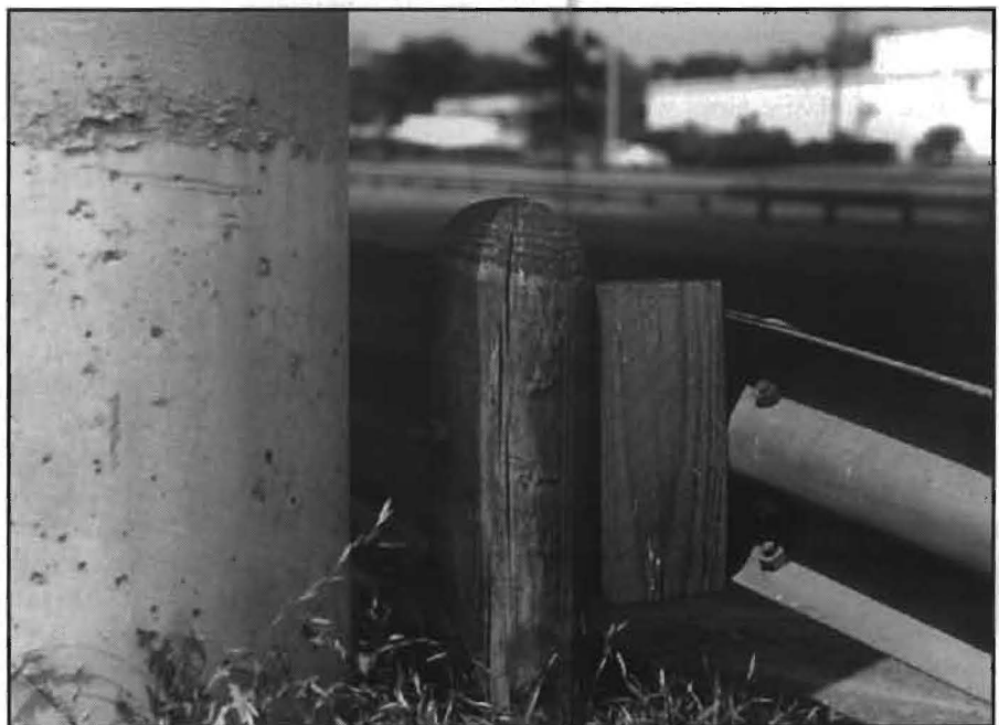
FIG. 4: Here a timber block carries the rail out over an unseen curb.
