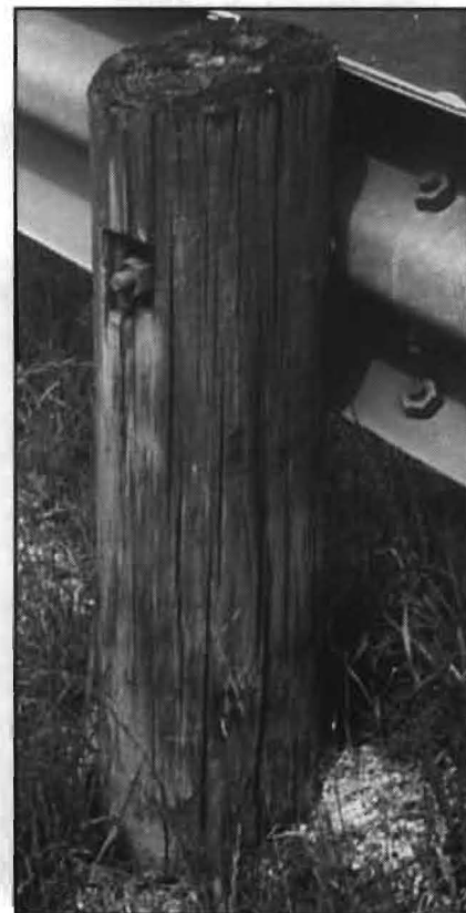
FIG. 3: Typical wooden post. The cracks seen here are not a structural problem. However, cracks expose untreated areas of wood and speed deterioration.
