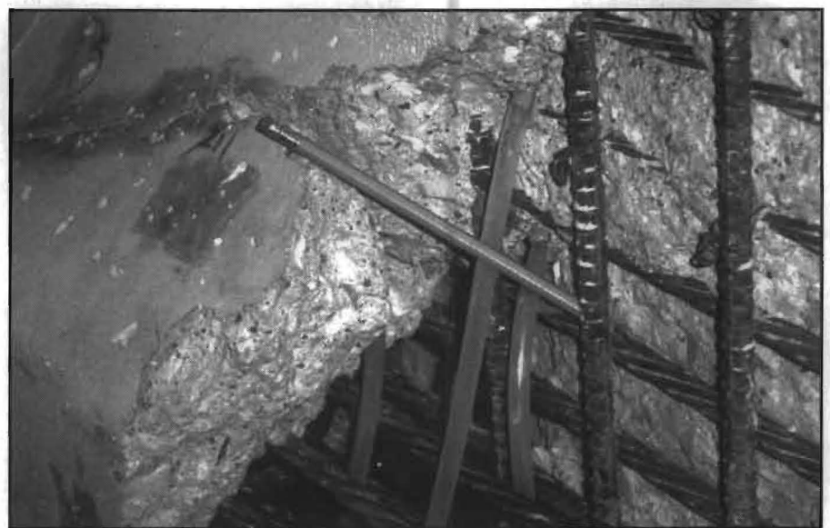
FIG. 6: Steck Ave. RR bridge beam showing epoxy injection tubes in place.
