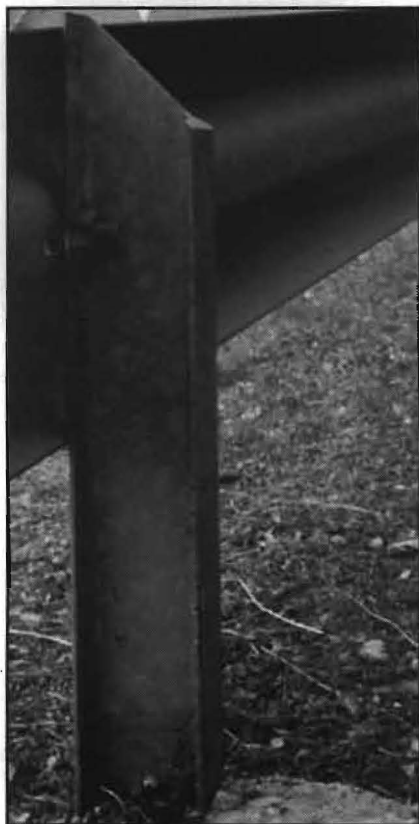
FIG. 2: Not-so-typical steel post. This variety is no longer in use, but when rails become obsolete, they remain in place until they need to be repaired. On this post, the grains from galvanizing are visible.
