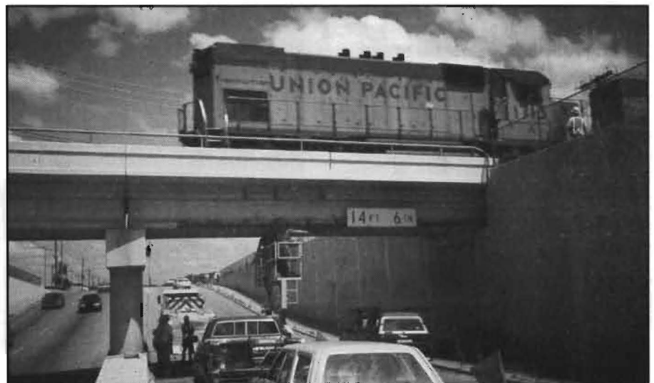
FIG. 1: The 0-1370 research team examines impact damage at the Steck Ave. RR bridge in Austin, TX.
