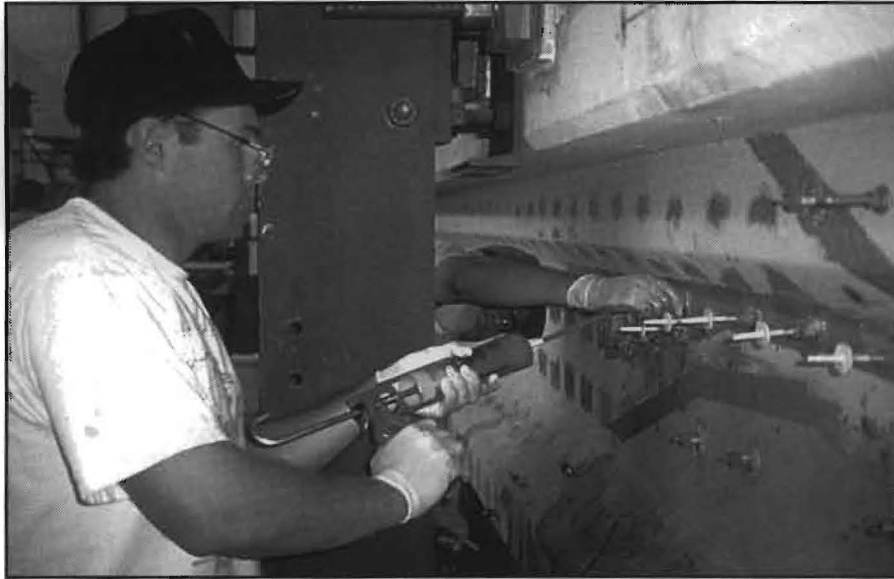
FIG. 7: Project 0-1370 graduate student uses hand-held, low-pressure caulking-type gun to inject epoxy into the Steck bridge beam.
