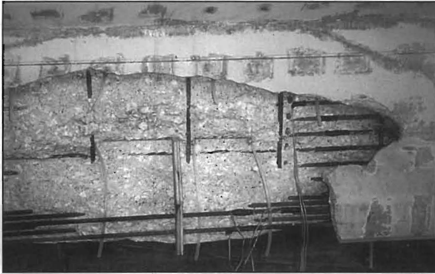
FIG. 4: The impact-damaged beam from the Steck Ave. RR bridge cleaned, sawed, and ready for patching material. This beam was removed to Ferguson Lab and instrumented for testing during Project 0-1370. Note plastic tubes shoved into cracks for future epoxy injection.
