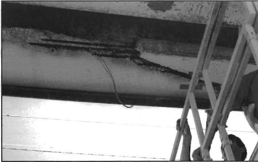
FIG. 2: Close-up of the damage to the Steck Ave. RR bridge. The traveling public must be protected from falling debris.
