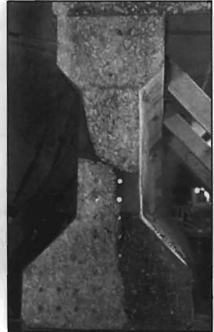
FIG. 8: Cross section of repaired Steck bridge beam. Different shades of gray denote different types of patching materials.
