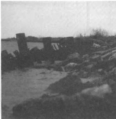
Undercut timber and rubble retaining wall along SH 82.
