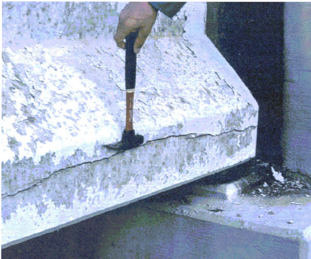
Typical premature concrete deterioration. Photo shows full-length horizontal cracks.
