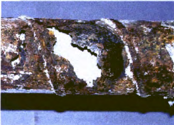
Corrosion of galvanized steel post tensioning duct
