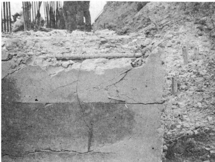
Fig. 10 End of foundation section which measured 24' long, 8½' wide and 2½' deep. Note distress cracks and lack of aggregate-paste bond. Scale is indicated by pocket knife.
