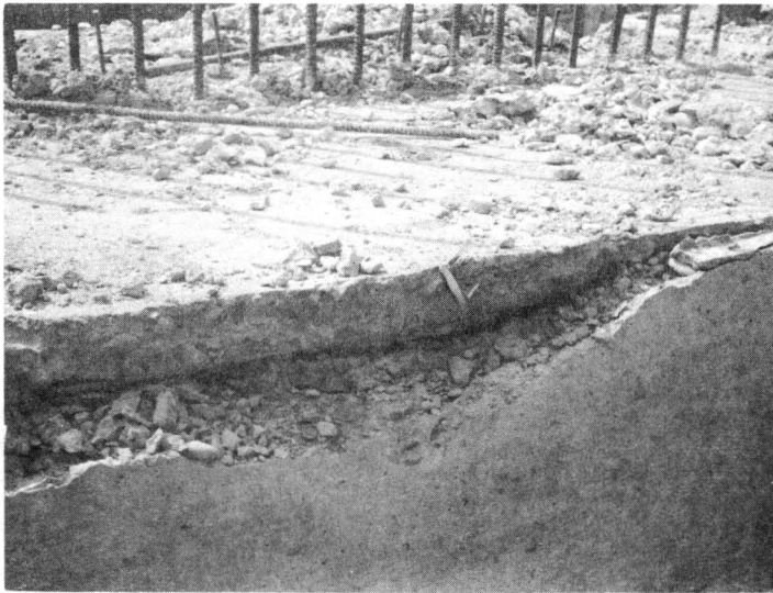
Fig. 9 View of retaining wall foundation before removal showing distress cracks. Scale is indicated by pocket knife.
