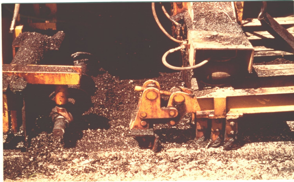
FIGURE 5 AUGERS LEVELING THE SURFACE AND MOVING SCARIFIED MATERIAL TOWARDS CENTER OF MACHINE
