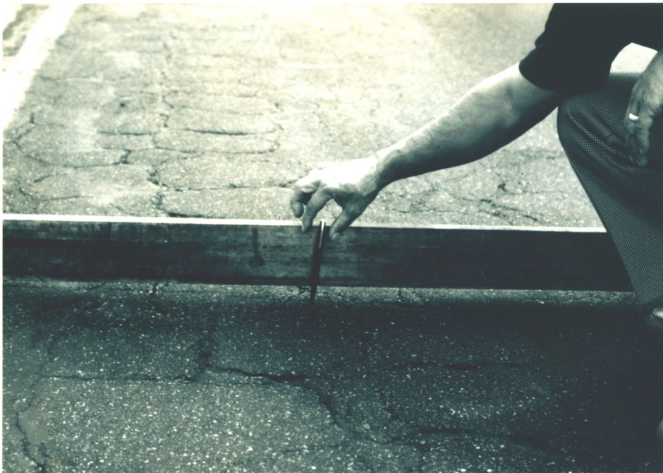
FIGURE 1 BADLY DEFORMED AND ALLIGATOR-CRACKED PAVEMENT
