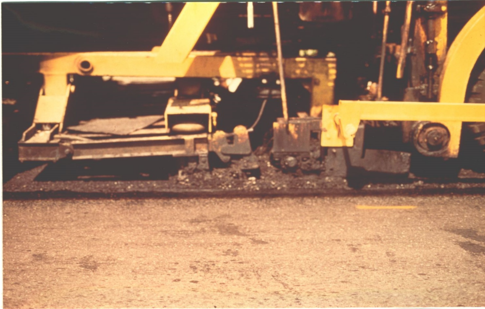
FIGURE 4 SCARIFYING OF EXISTING PAVEMENT SURFACE (Note air bag located above scarifying teeth. The air pressure in the bag controls the depth of the scarification.)
