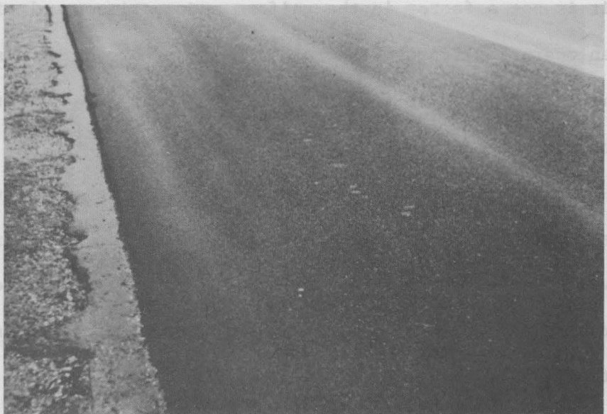
Figure 10. Photographed during rain of about \frac{1}{2} -inch per hour. Water is draining through the mat and out the edge of the surfacing.
