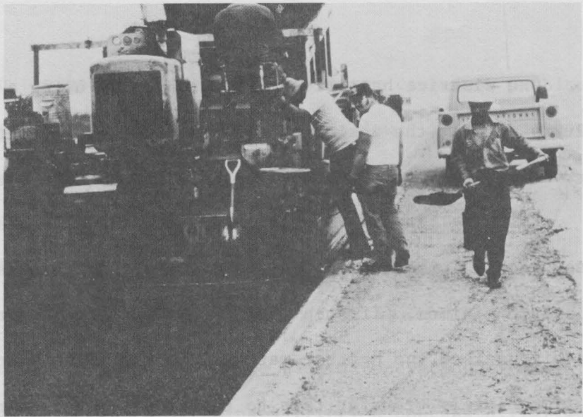
Figure 8a. Hot material is rapidly transferred to the area to be patched.
