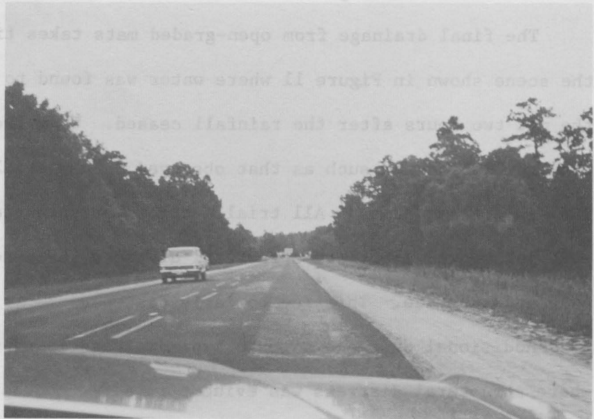
Figure 12. Entry of water causes early structural distress in East Texas pavement.
