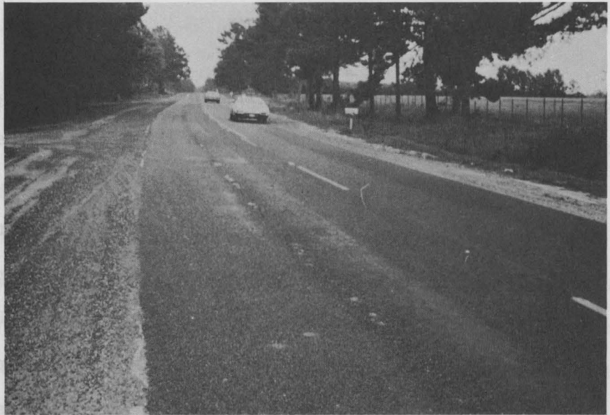
Figure 16a. A dragging screed causes aggregate crushing and raveling between wheel-paths where overlay is too thin.
