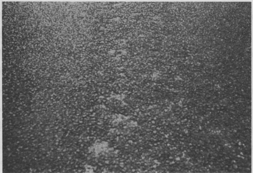
Figure 16b. Close-up of damaged area.
