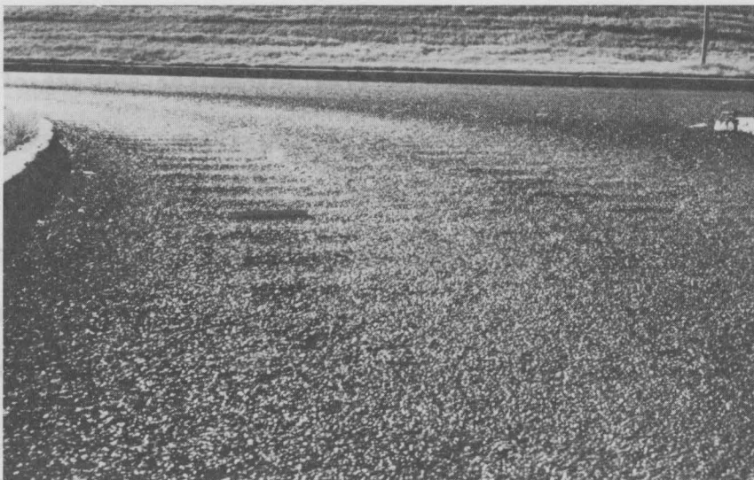
Figure 5. Plastic instability of "open" graded thin overlay.
