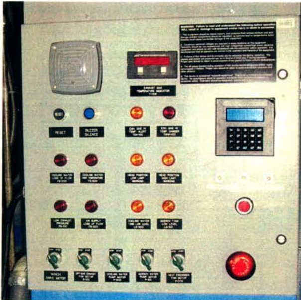
Figure 8. Interlock and Warning Panel
