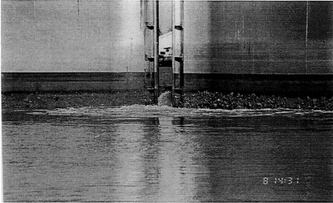
Figure E-15. Opening of gates at the East Lock (note approx. 1 ft difference in water level).
