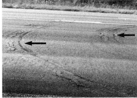
Early traffic can cause damage.
