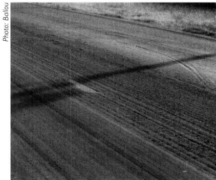
Excessive drag marks and scratches
