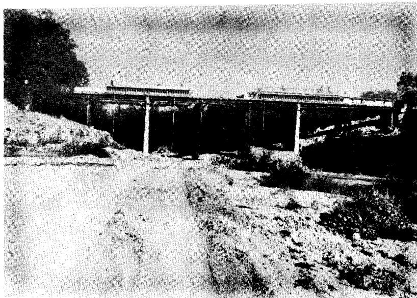
Existing piers are visible in picture at extreme right and extreme left (in trees.) The two intermediate piers are new construction required to complete the sub-structure to support the special design 198 ft. 4 in. concrete girder unit (59 ft. 2 in. -80 ft. -59 ft. 2 in.) Steel piling shown in picture are false work.
