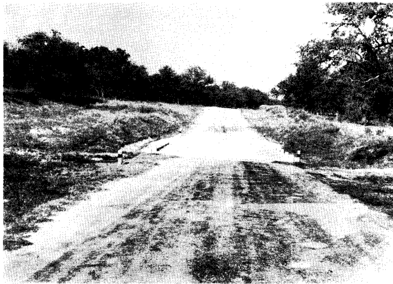
Overflow type structure. 3-5 ft. x 3 ft. x 26 ft. MBC-1 Mod. 45 deg. skew. 25 ft. Class "B" Concrete approach slabs. This structure is located in extremely sandy soil. This structure was recently subjected to overflow due to unusually heavy local rains.
