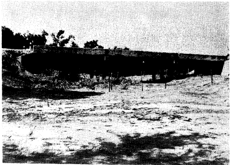
Standard 25 ft. (FS-8-20-25) end spans required modification in order for slab to bear on abutment wings. Note how curbs have been extended to rest on the angled section of the existing abutment wing.
