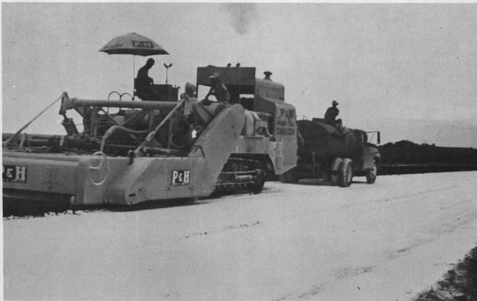
Photograph No. 21, similar to No. 20 except note water truck in front of P&H mixer.
