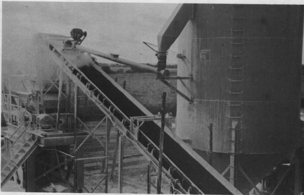
Photograph No. 17, Note lime being added to conveyor belt carrying gravel and soil binder.
