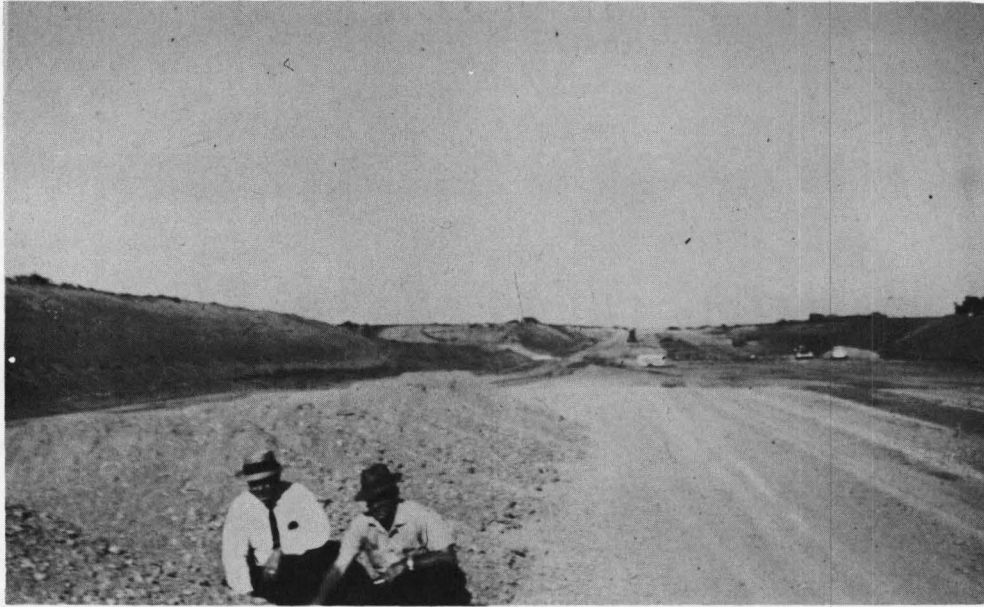
Photograph No. 22. Covering of lime stabilized subgrade with gravel subbase material promptly after curing 7 days.
