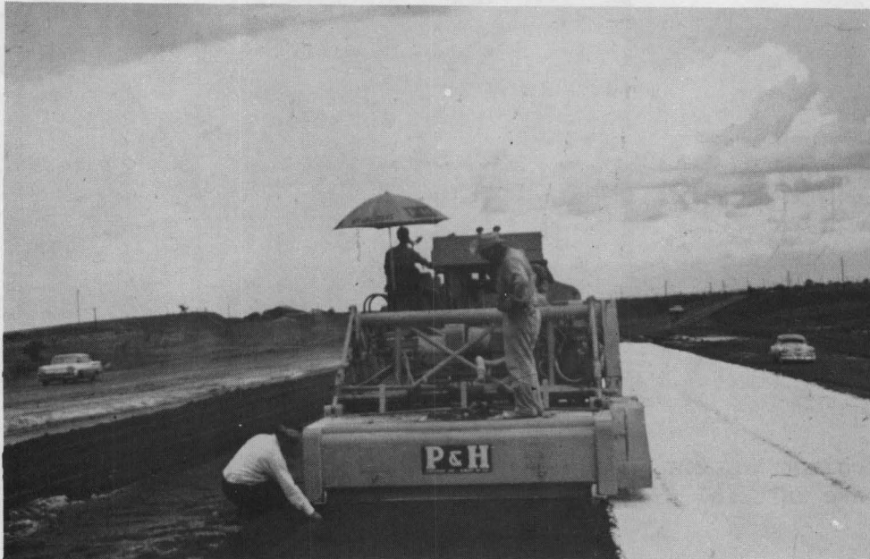
Photograph No. 20, showing lime and water being added to plastic red Vernon clay with a P&H mixing machine.
