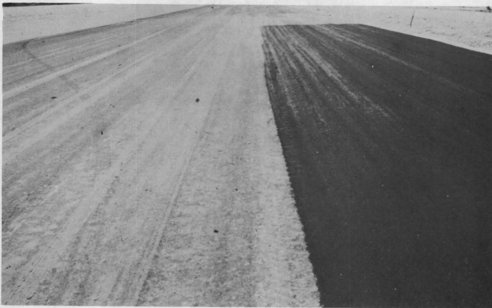
Photograph No. 28. Clay-lime subgrade cured by sealing with MC-1 at left (note penetration) and asphaltic emulsion at right. It was decided to place sand-shell subbase material on clay-lime at an early date instead of trying to seal with asphalt.
