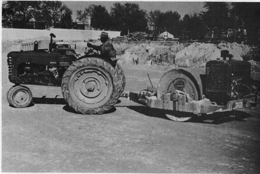
Photograph No. 11 Compacting crushed rock fill to specified density with vibratory roller.
