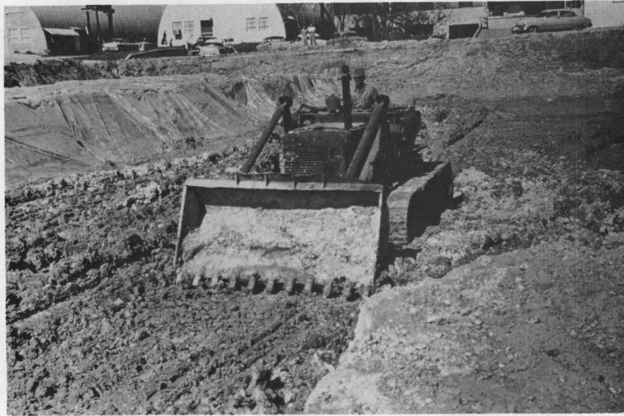
Photograph No. 7 Mixing lime into soft subgrade with bucket teeth of front end loader.
