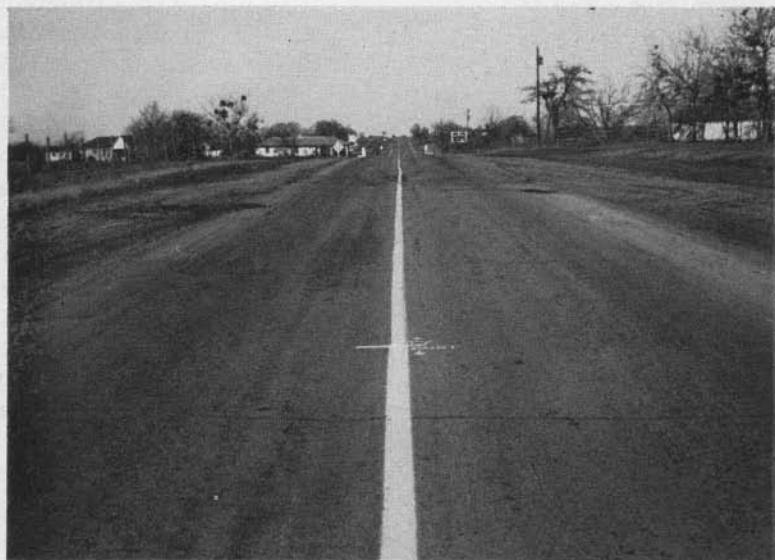
The hot-melt plastic stripe used for a white center line on an asphaltic concrete pavement. The horizontal chalk line shows the end of a 3-month-old paint stripe in the foreground with the hot-melt plastic stripe in the background.
