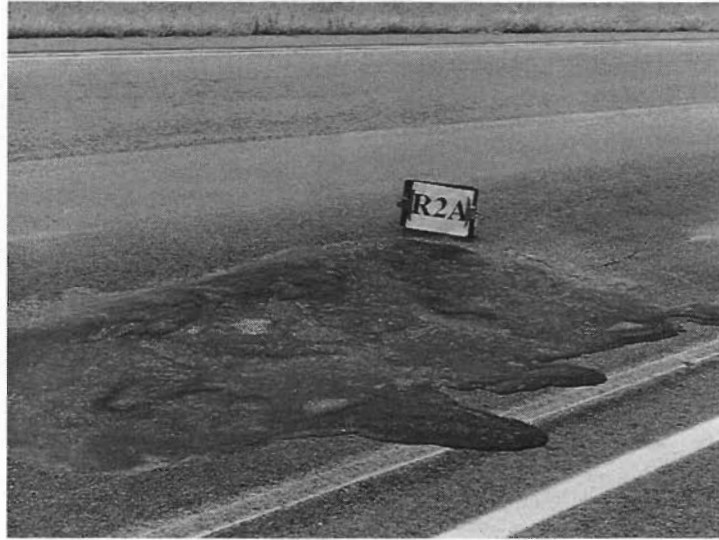
Figure 2.4 Example of failure in R2A
