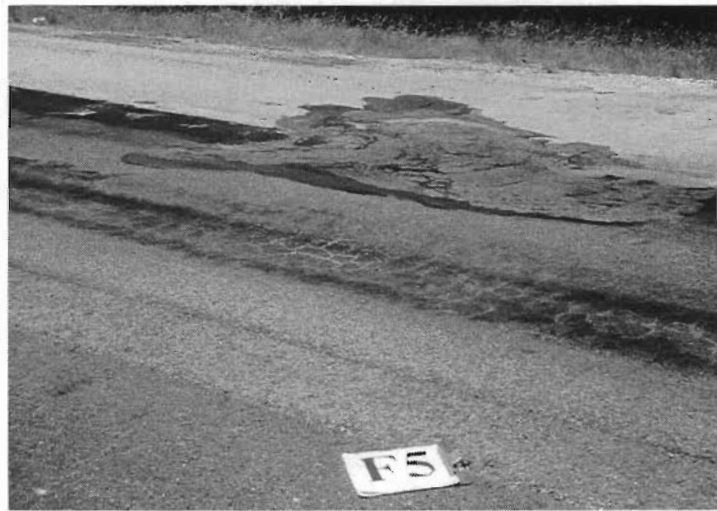
Figure 2.5 Example of failure in F5
