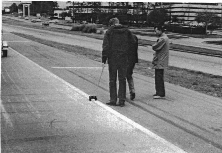
Fig 3.2. CTR personnel are conducting condition survey on the 10 test sections, IH 610 North, Houston.
