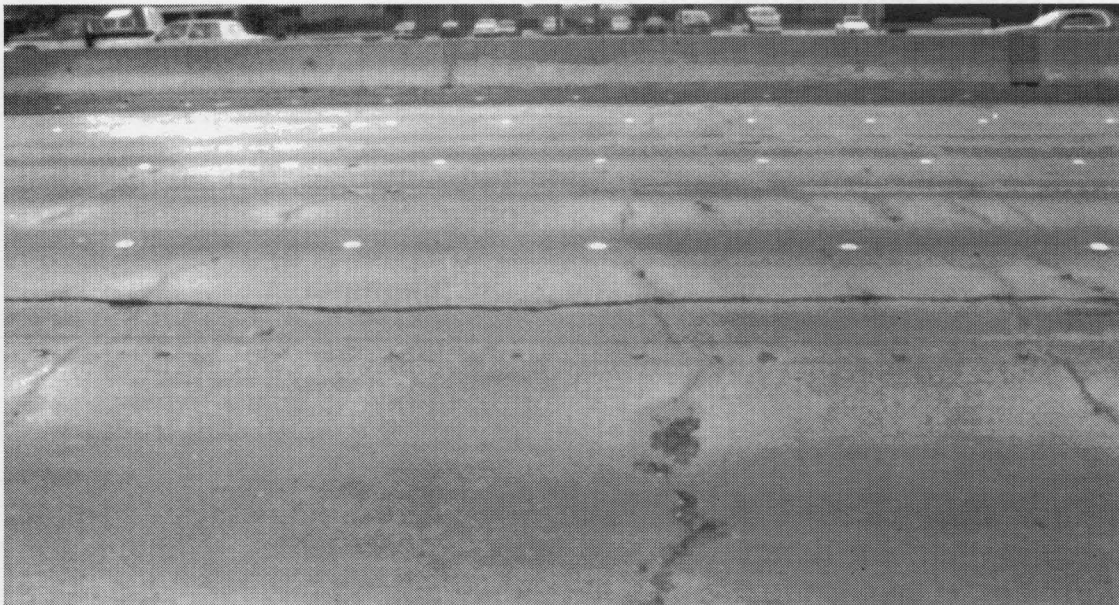
Figure 1. Loop 610 before overlay. Note longitudinal cracking and surface spalling.
