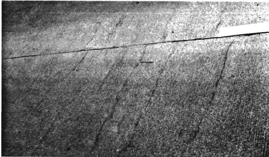
A portion of the IH-610 thin bonded overlay test section with evident lateral cracks.
