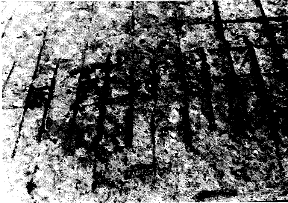
Figure III.2 Condition of delaminated area after milling
