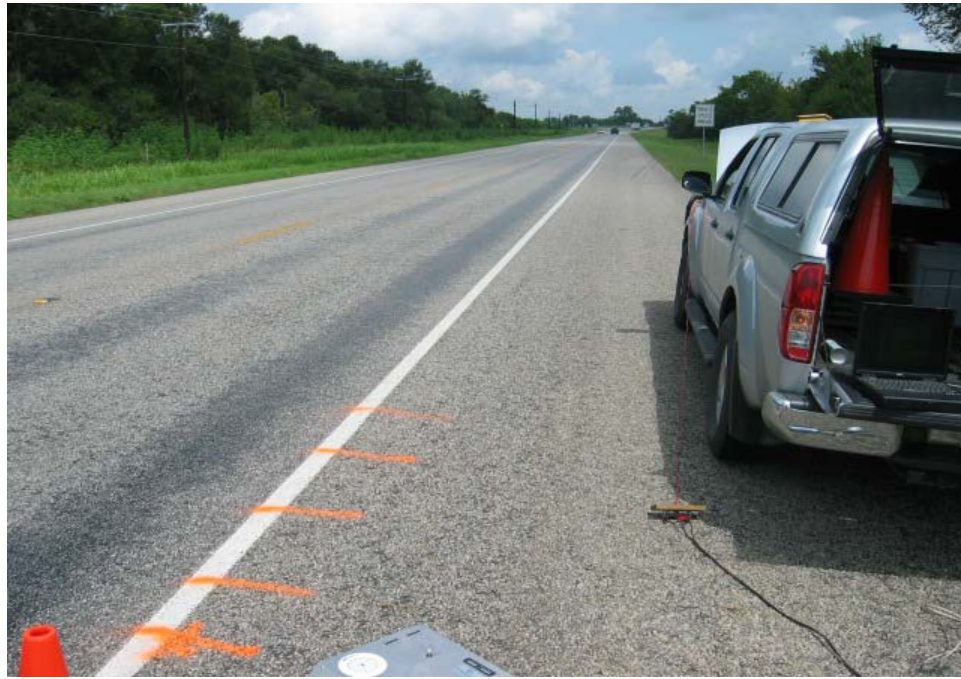
Figure A.3 Seal coat with excessive flushing
