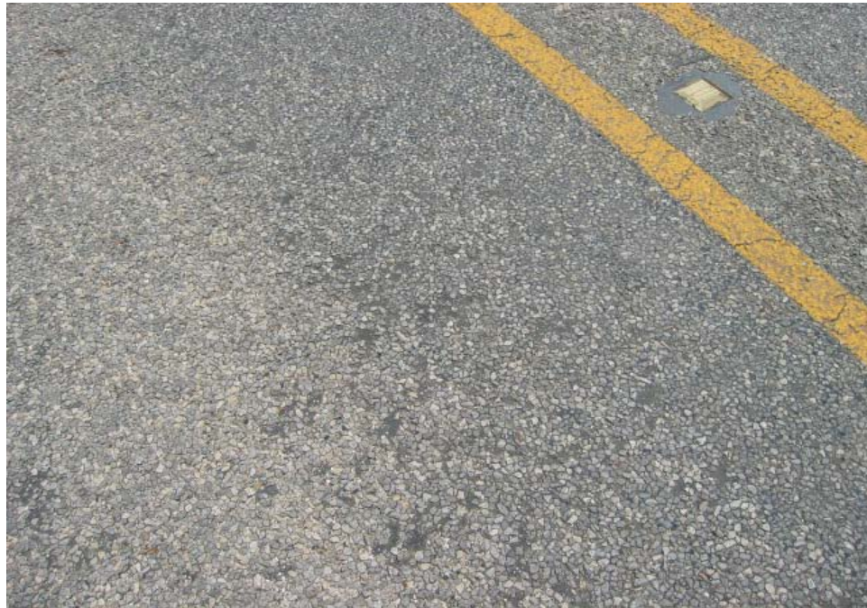
Figure A.8. Close up of seal coat showing little distress
