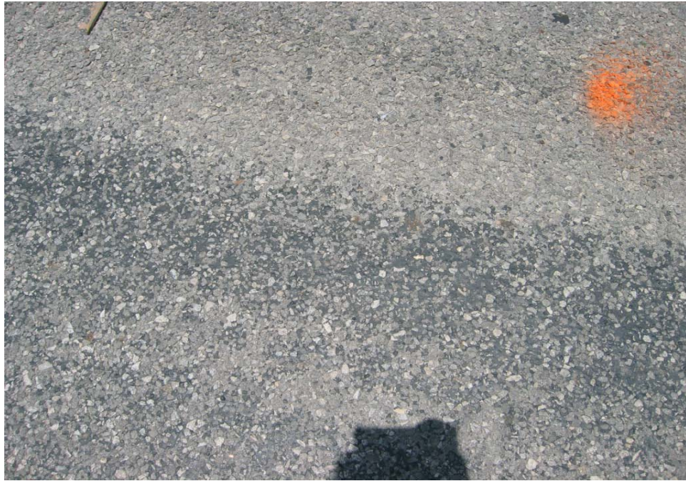
Figure A.6 Close up of seal coat with moderate flushing
