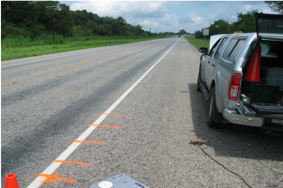
Figure 1.1. Seal coat pavement showing signs of flushing
