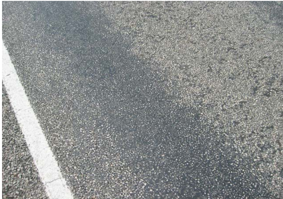
Figure A.4 Close up of seal coat with excessive flushing
