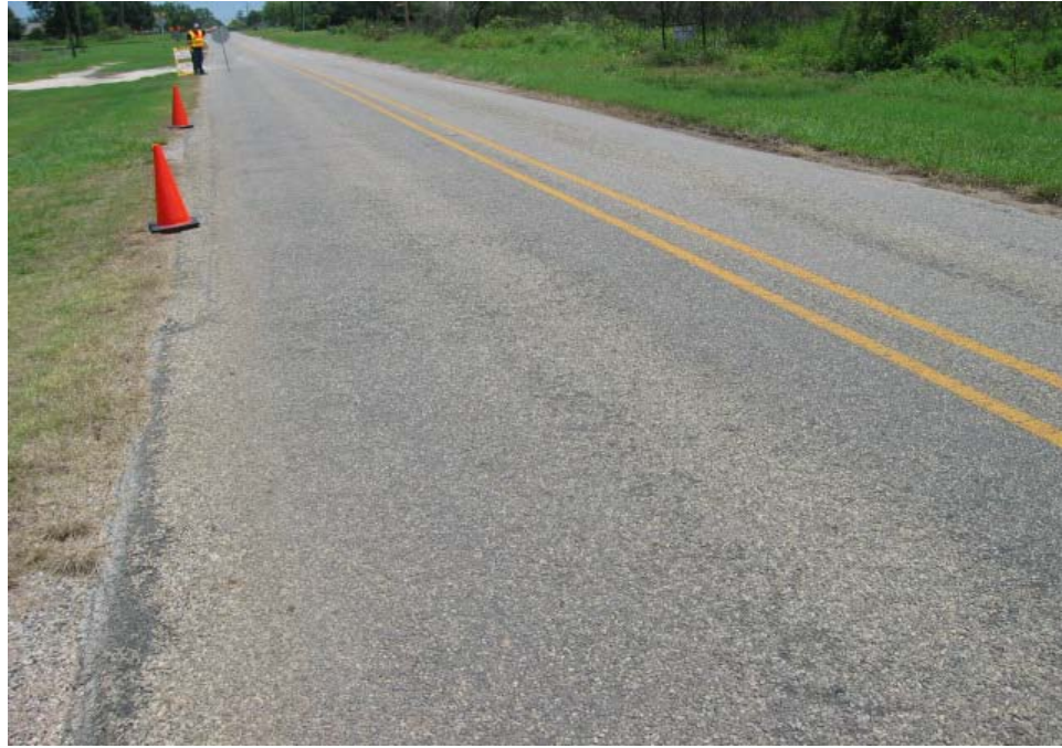
Figure A.7 Seal coat showing little distress
