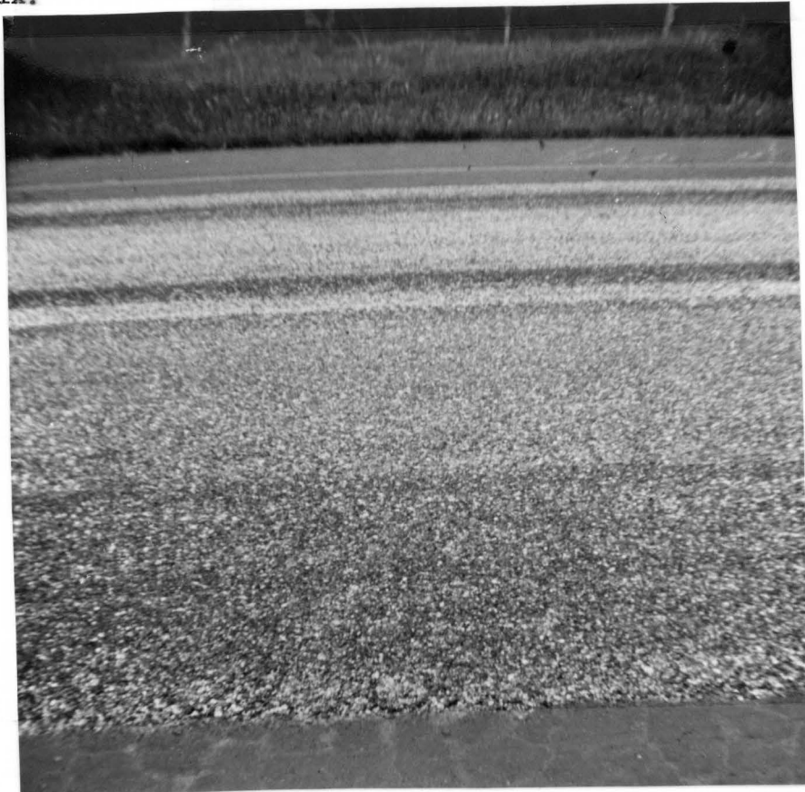
Same section as Photo 38, with asphalt rubber seal coat in place. Note cracks showing through sand asphalt mixture.
