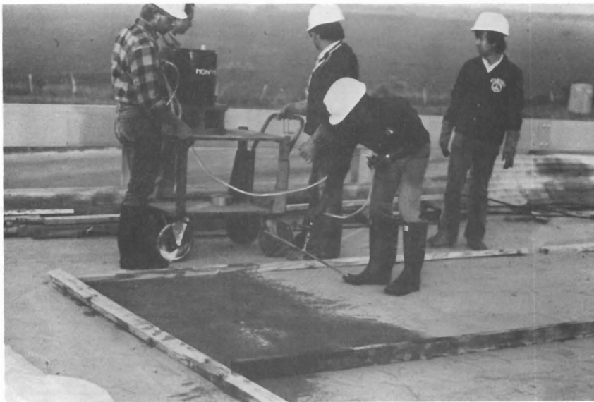
Figure 17 - Monomer Application Equipment
