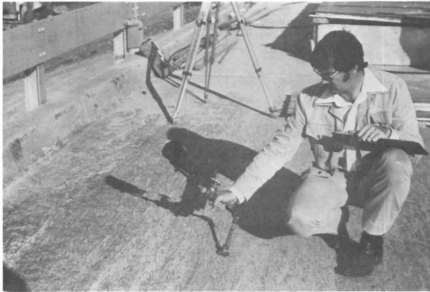
Figure 6 - Burner Used for Drying Operation
