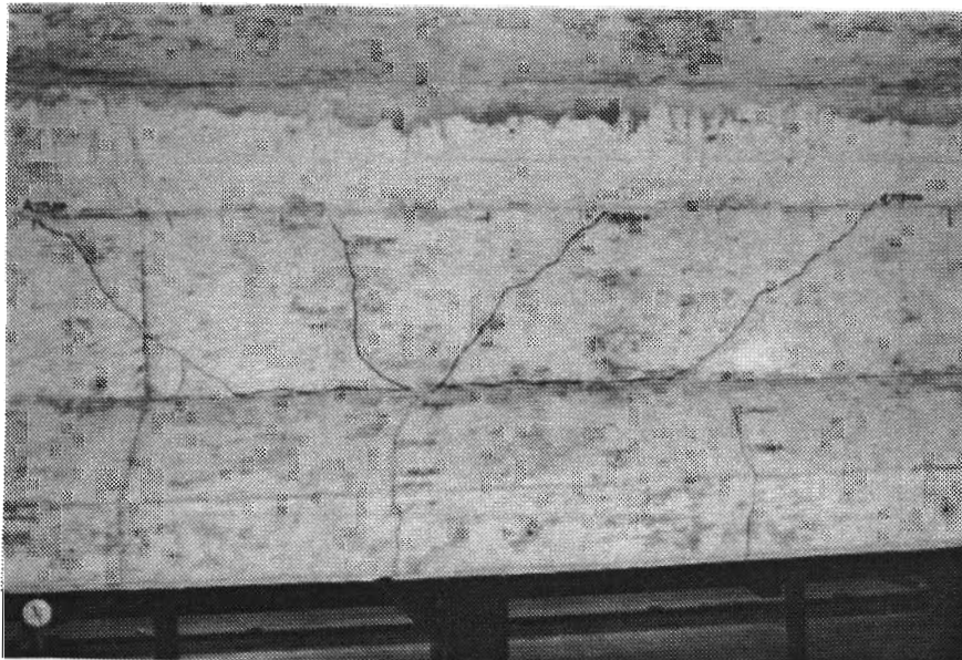
Fig. 4.38 East side (top) and west side (bottom) torsional cracking observed in the flexural failure zone
