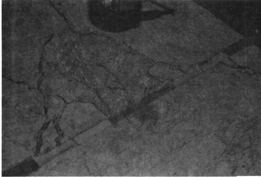
(a) Before repair.
