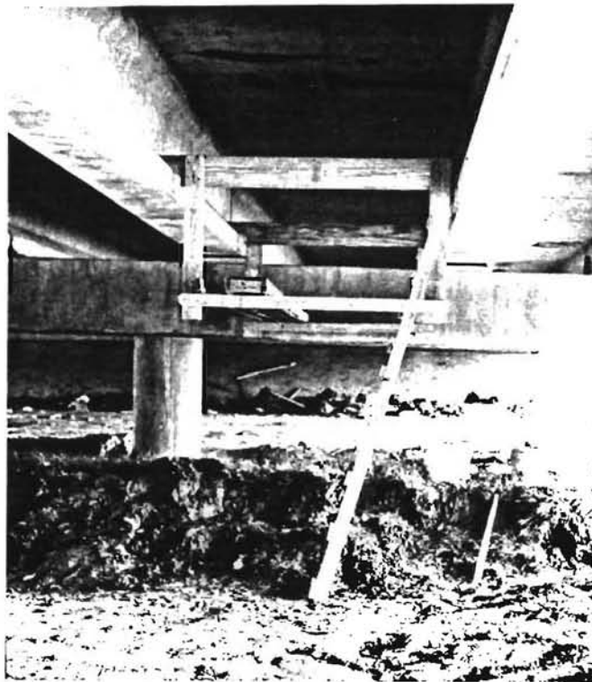
Fig. 2.6 Platform used to reach bottom surface of slab at east end of bridge for instrumentation application
