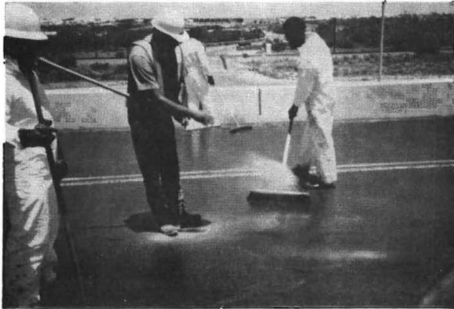
Fig. 5.25 Pouring Sand Onto the Slab in order to Restore the Surface Skid Resistance of the Concrete Topping.
