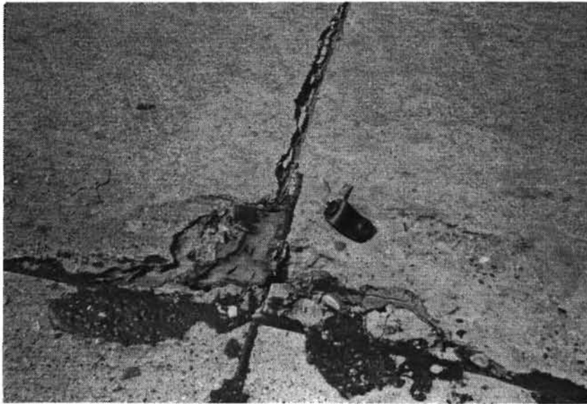
Fig. 7.1 Debonding of a Joint at a Large, Sealed Spall
