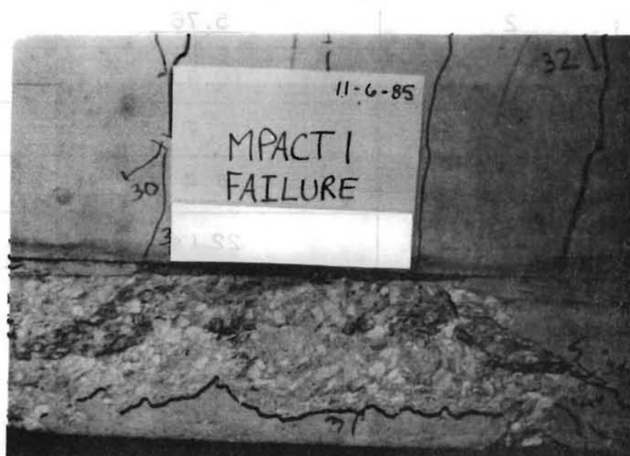
Fig. 4.21 Slab shearing failure: MPACT1
