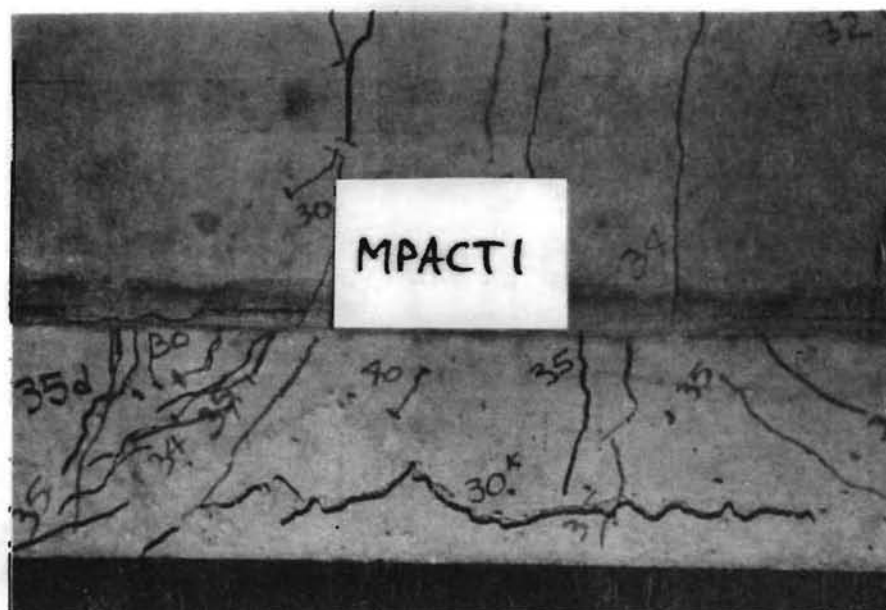
Fig. 4.20 Initial slab shearing crack: MPACT1
