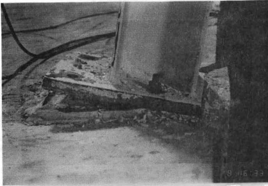
Fig. 5.61 East-end post location at failure
