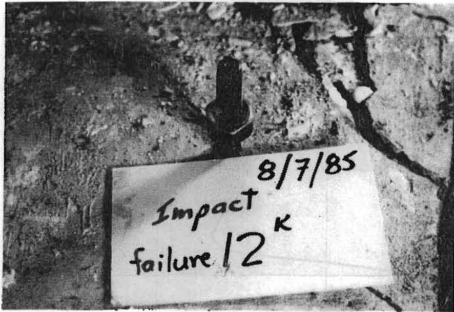
Fig. 5.33 Fractured tension anchor at west-end post
