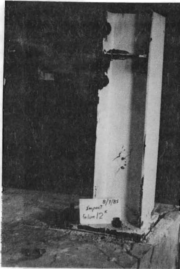
Fig. 5.32 Fracture of tension anchor at west-end post
