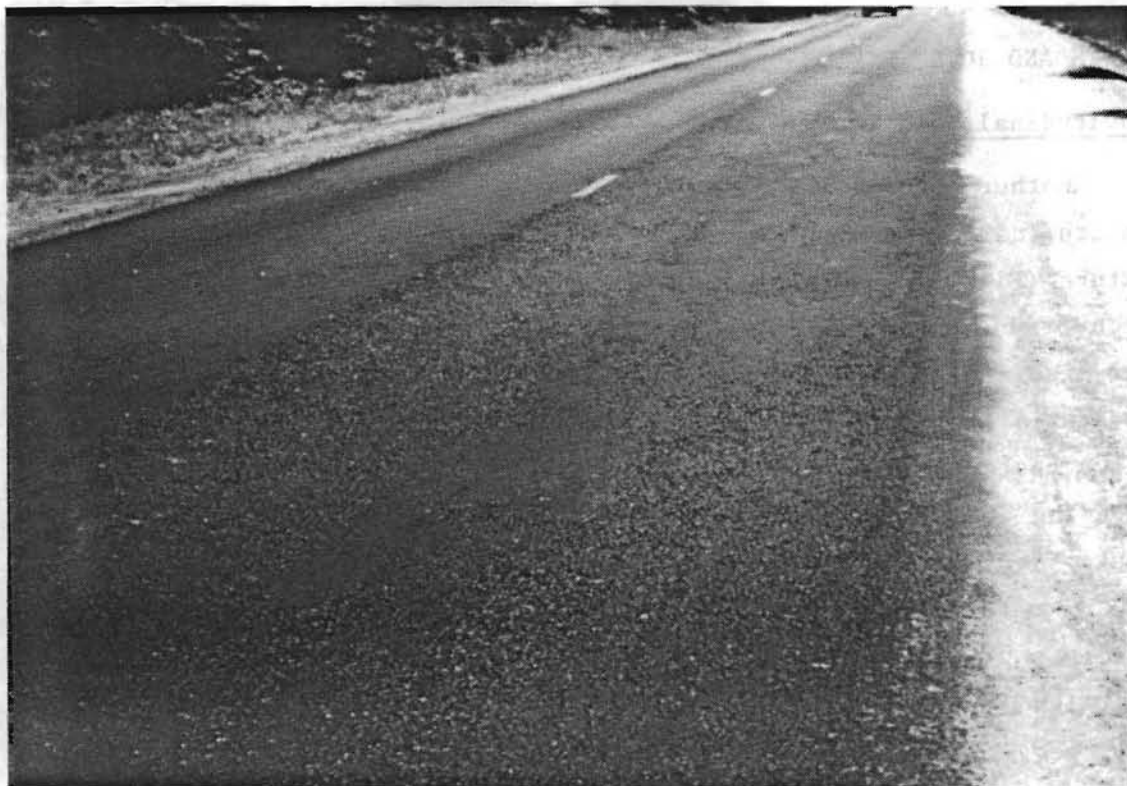
Figure 5.5. Severe segregation resulting from starving of augers, visible as coarse areas near edge of mat
