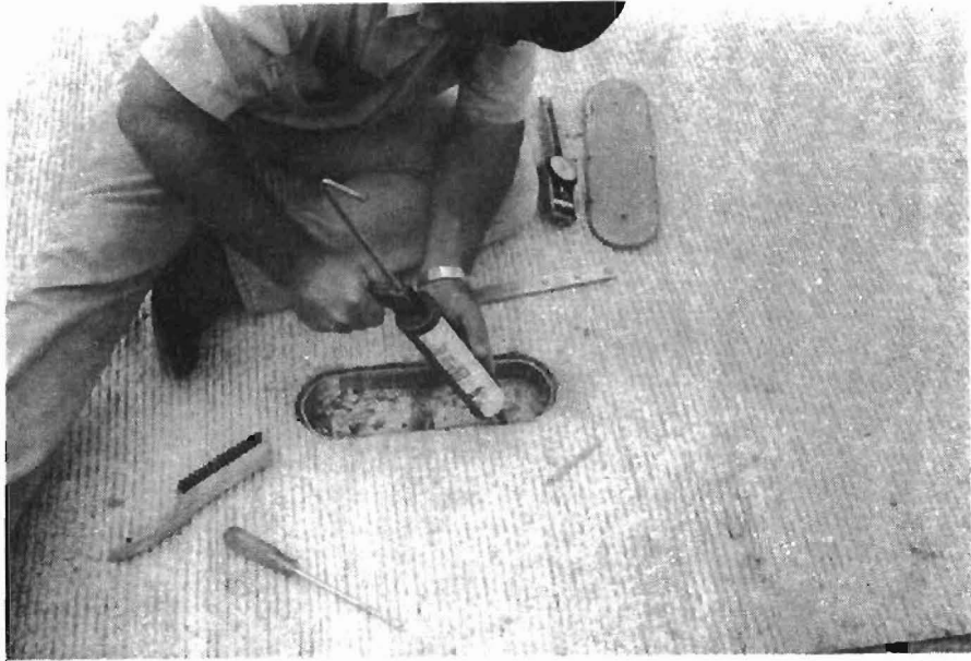
Fig 3.7 . Installation of inside gauge plugs; sealing bottom of a measurement box with silicone compound.
