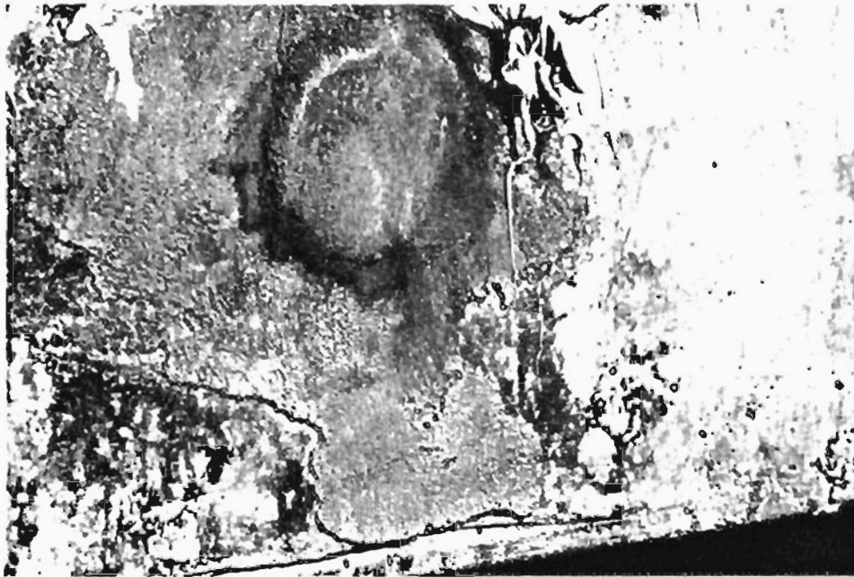
Fig. 4.8 ° Discoloration of mortar anchorage plug in some areas after prolonged exposure
