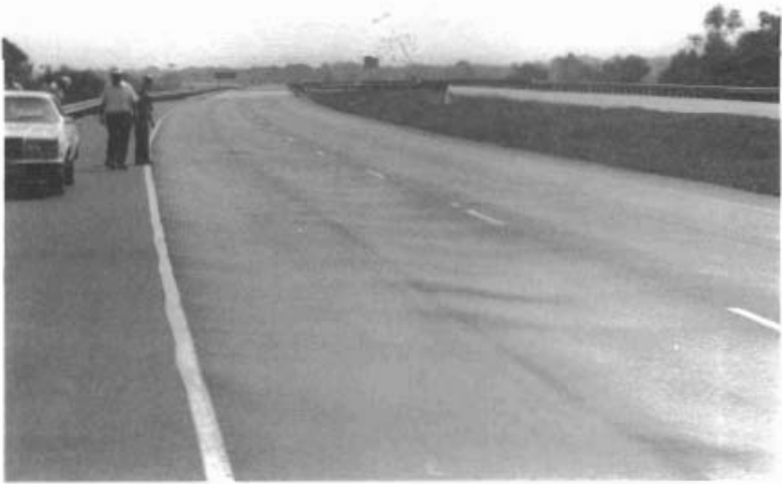
Fig 1. Typical rutting and corrugation distress occurring on IH-10, Columbus.
