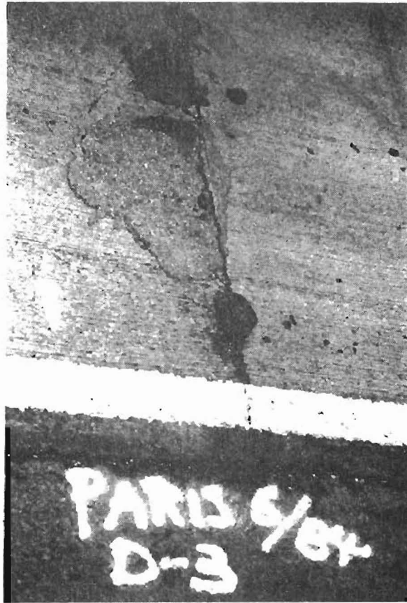
Fig. 7.13. Spall Area Before Repair
