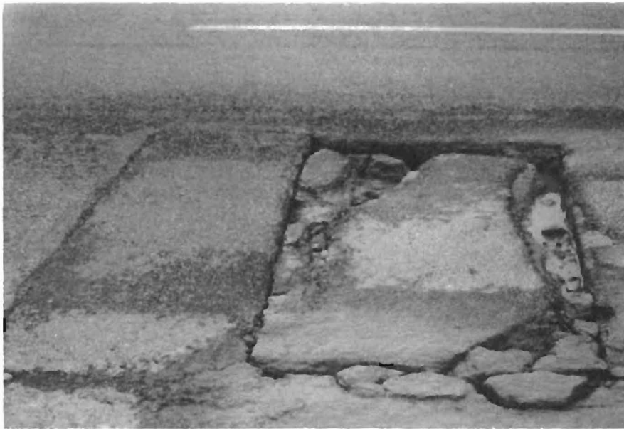
Fig. 6.9. Condition of Repair No. AMA-HS Before Being Repaired.
