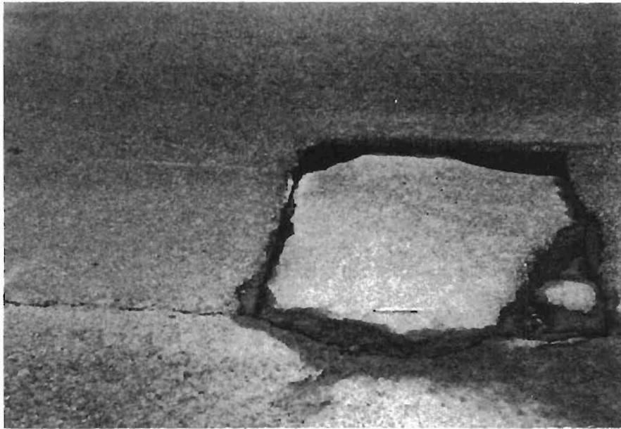
Fig. 6.6. Condition of Repair No. AMA-DCI Before Being Repaired.
