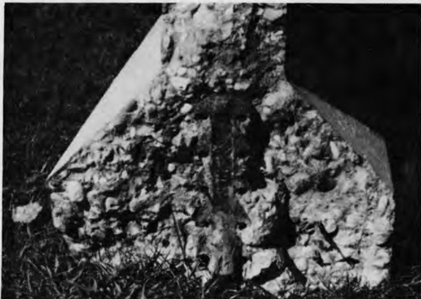
Fig. 4.65 Drape hardware at the failure crack.
