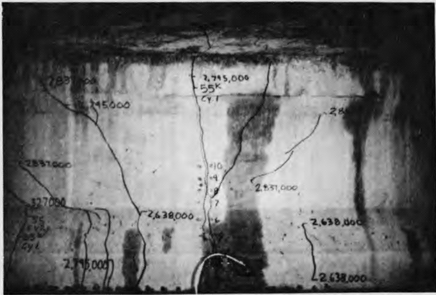
Fig. 4.64 Flexural cracking prior to the static ultimate test
