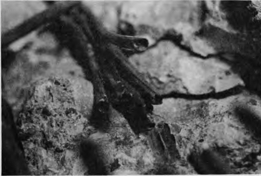
Fig. 3.41 Beam specimen wire fatigue fractures
