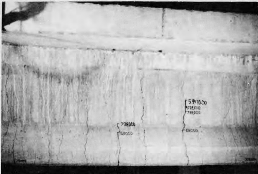
Fig. 4.85 Flexural cracking on the east side of Specimen A-22-NP-3.5-OL-5.95 (NF) after ultimate testing
