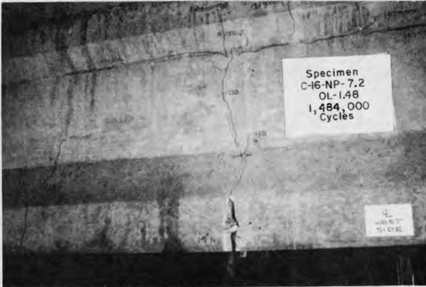
Fig. 4.14 Concrete spalling at 1.484 million cycles
