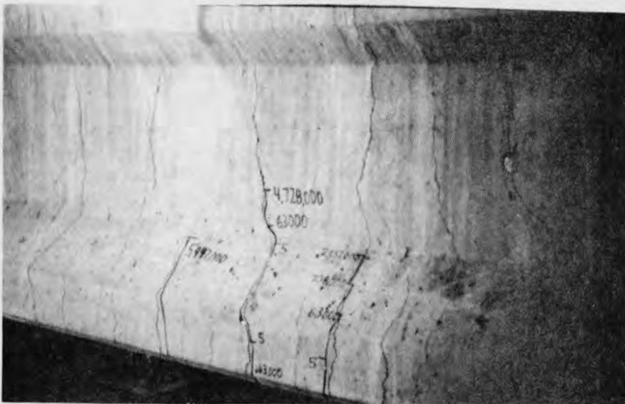
Fig. 4.86 Flexural cracking on the west side of Specimen A-22-NP-3.5-OL-5.95 (NF) after ultimate testing
