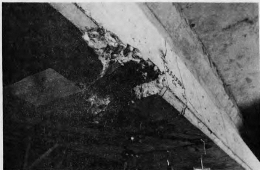
Fig. 4.50 Concrete spalling on the west side of the specimen which occurred at 3.19 million cycles
