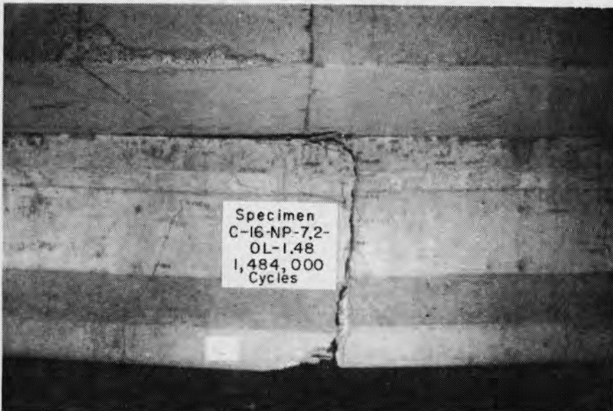
Fig. 4.15 Cracking after static ultimate test
