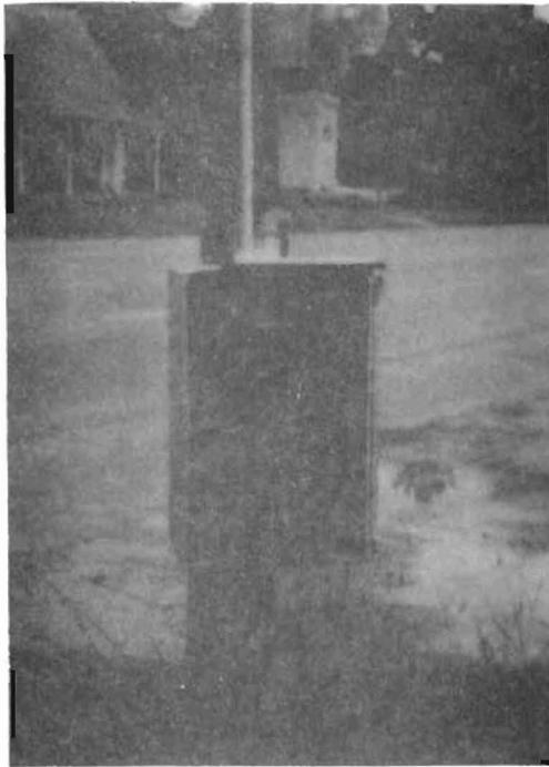
Speed Analysis System And Flasher Controller
