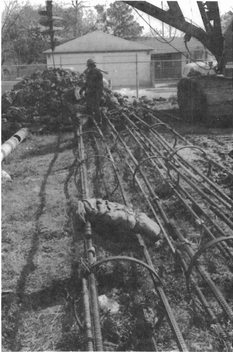
Fig. 5.15. Soil inclusion (1/2 cross-sectional area) attached to steel reinforcing cage prior to installation.
