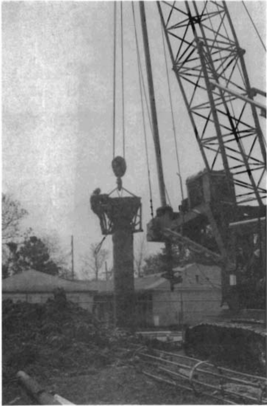
Fig. 5.22. Placing concrete in upper portion of pier by partially removing steel casing and utilizing concrete bucket.
