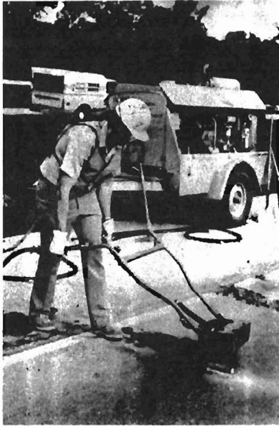
Fig. 4.10 Opening (Chasing) Cracks.
