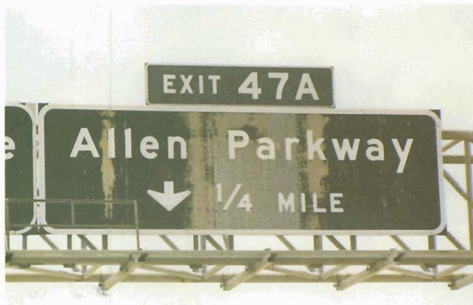
8 years Field Service - The release agent on plastic coated plywood substrate caused delamination. Coating delaminated after 5 years.
